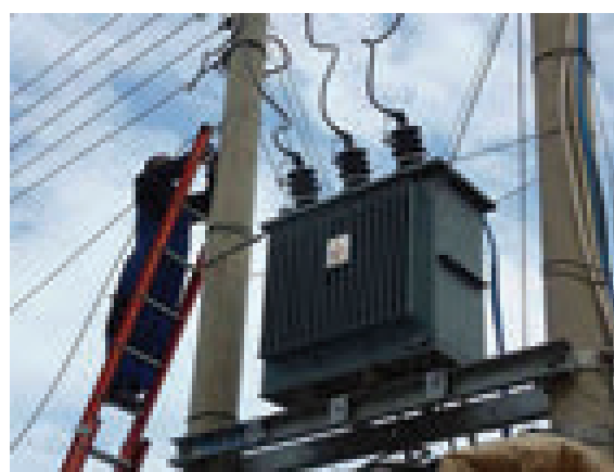
Figure 4.32(b) Roadside transformer
