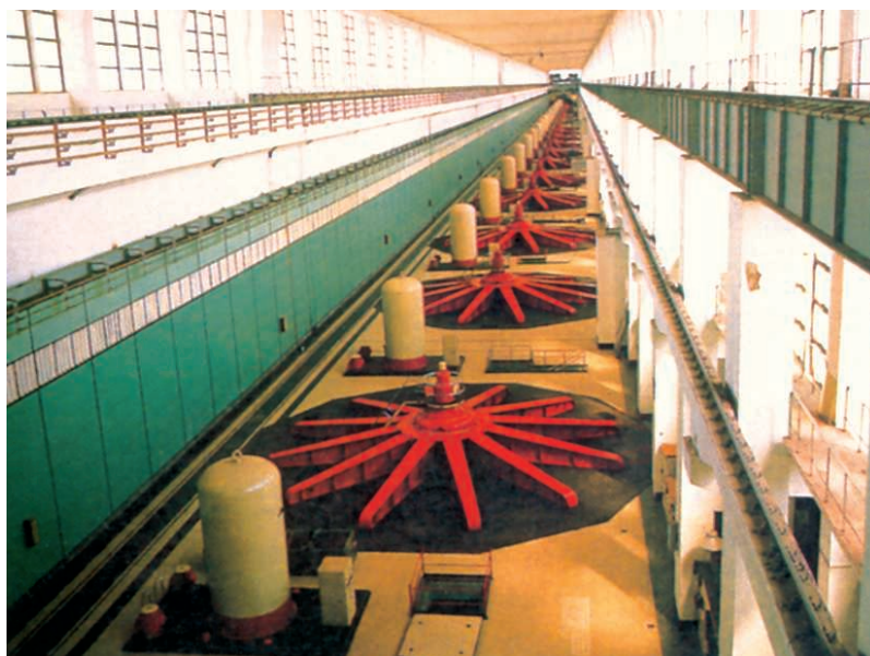
Figure 51. This photograph shows a number of turbines in a hydroelectric power house (or hydroelectric power station). The fast flowing water coming from the dam reservoir, rotates these turbines rapidly. The rotating turbines then rotate the electromagnet of the electric generator (called alternator). When the electromagnet turns rapidly inside the huge fixed coil of generator, then electric current (or electricity) is produced by the process of electromagnetic induction.
